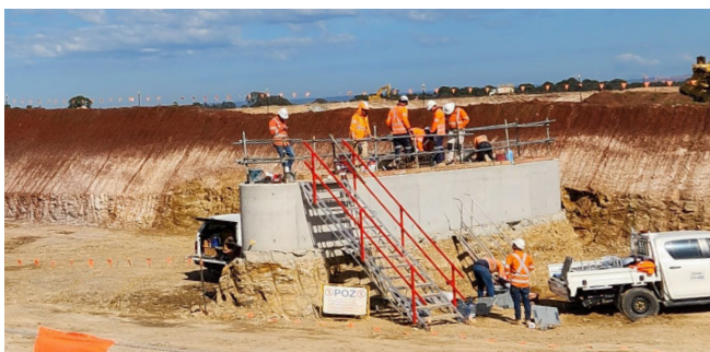
Headstock Access - SCAW Project
